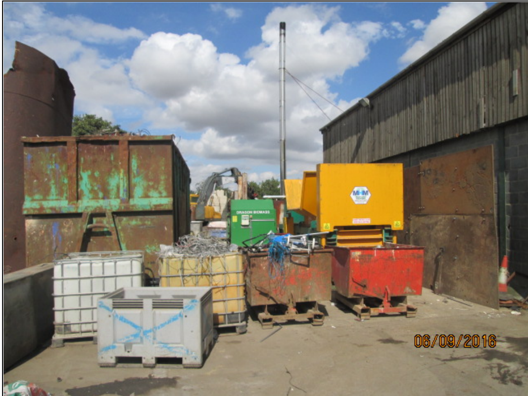
View of Biomass Boiler and flue from within scrapyard/waste recycling facility.
